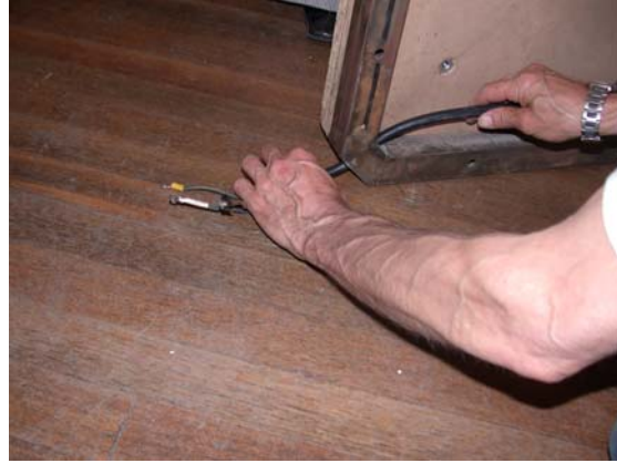
At the centre of the floor plate the cable is pulled upwards
