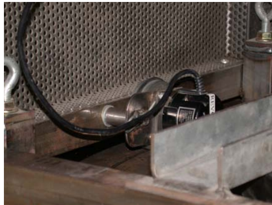
Tracking wheel/optical encoder is being connected to the inner left side of the frame.
