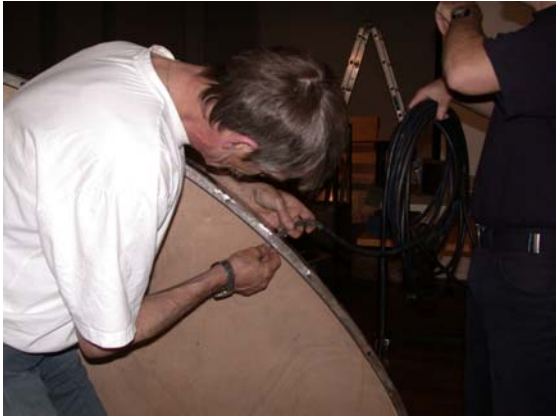
The power cable is being passed to the bottom of the floor plate.
